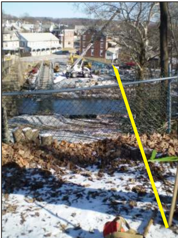
The pedestrian walkway is located to the south of the bridge construction. In photos the yellow line represents the placement of the walk.
